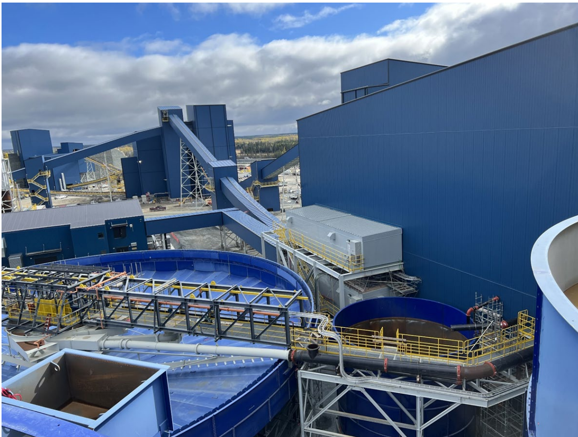
Pre-leach thickener, process plant and conveyors
