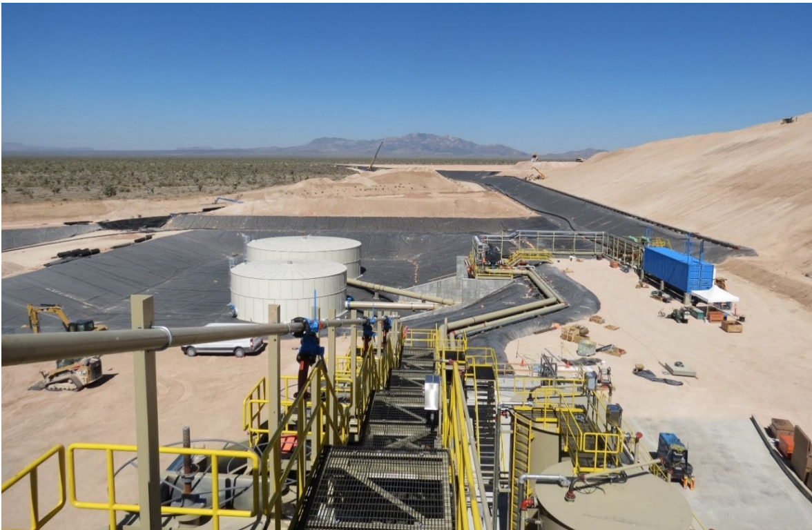
Figure 5 - Barren and pregnant solution tanks and containment area
