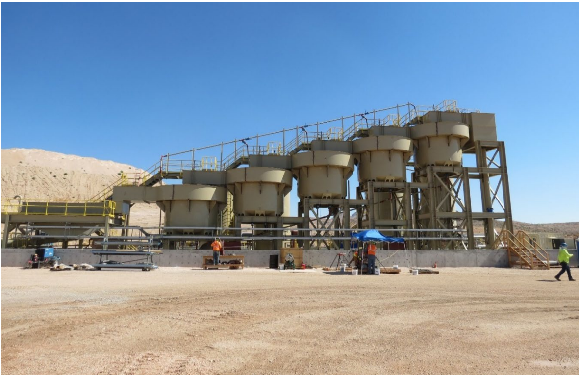
Figure 4 - New carbon-in-columns plant
