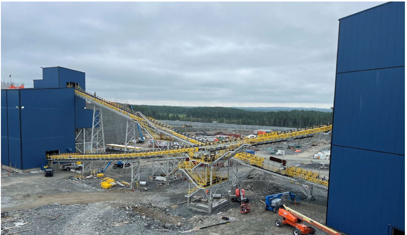
Conveyors between crusher and HPGR buildings
